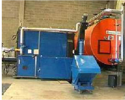
Figure 6. Burner and boiler of the Molins Energia plant [7]
