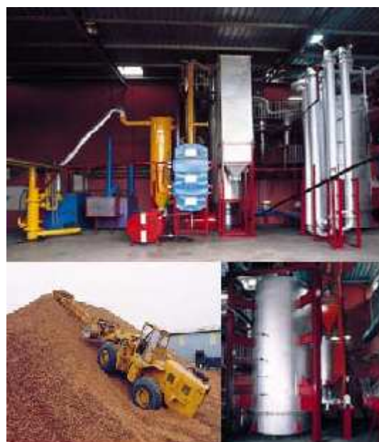
Figure 8. Biomass gasification plant in Mora la Nova (Catalonia) [8].
